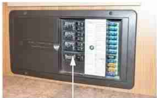
120-Volt Circuit Breakers -Typical View
