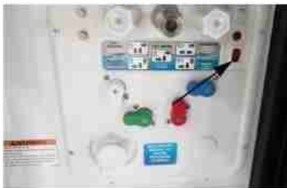
Water Center Panel service light -Typical View
