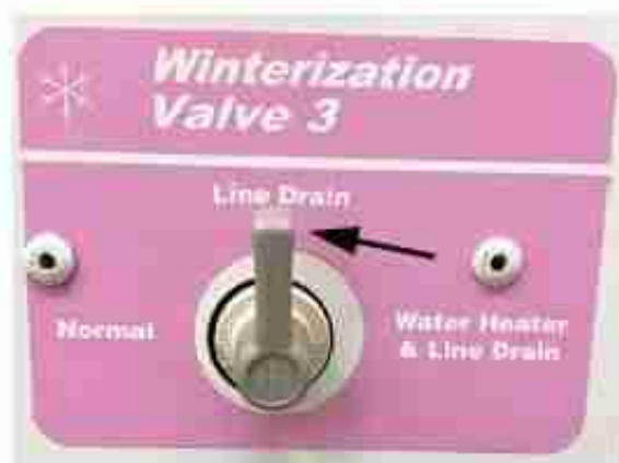
Winterization valve in the "Line drain" position. -Typical View
