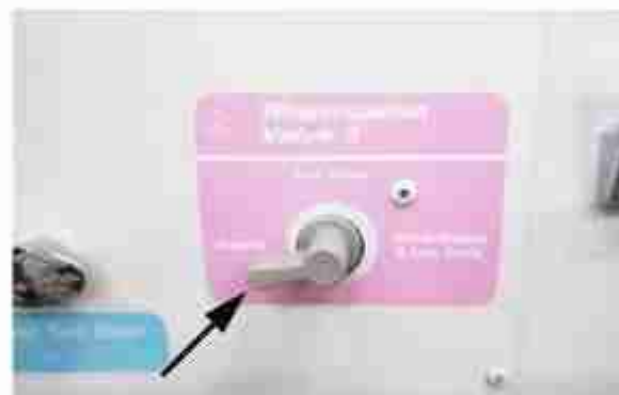
Winterization Valve 3 turned to the "Normal" position.
