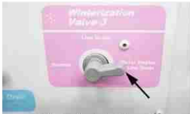
Winterization Valve 3 turned to the "Water Heater and Line Drain" position.
