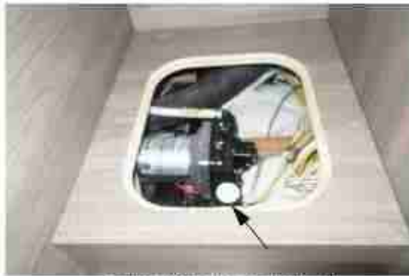
• The water pump strainer is located closest to the inside -Typical View
